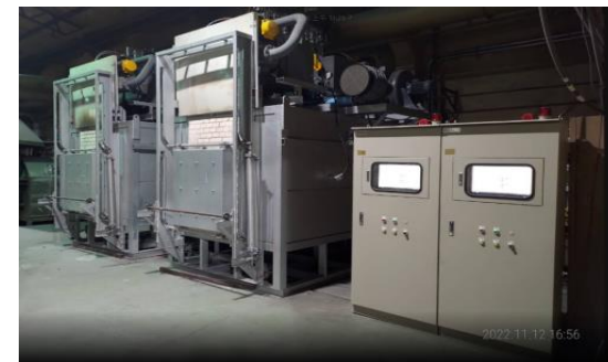
建置蓄熱式燒結爐
