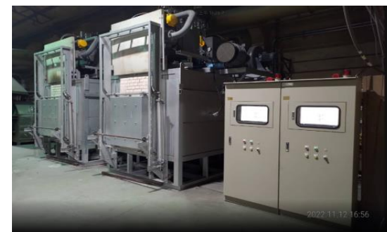
建置蓄熱式燒結爐
